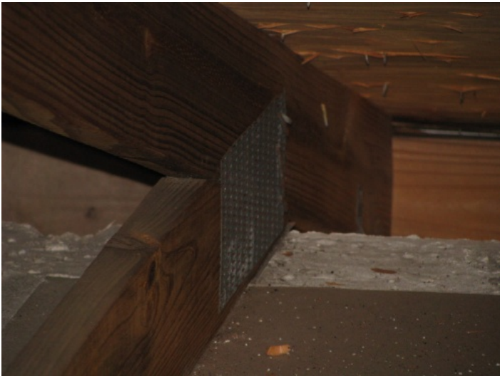
Roof to Wall Connection - strap not wrapped on back side
